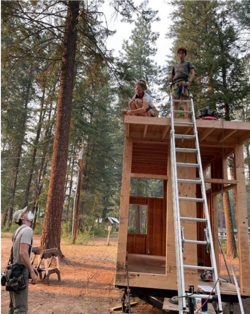
Cast Architecture provided plans for the compact dwellings, and the family of four constructed them with the help of family and friends.
