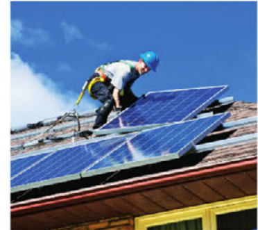
▲ Even as far north as sub-Arctic Alaska, solar panels are viable energy generators.
